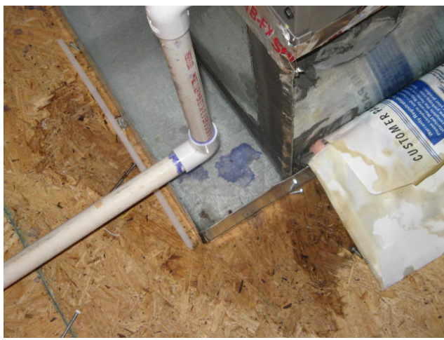
OVERFLOW DRAIN PIPING TO FURNACE FILLED WITH WATER
