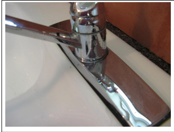
MINOR LEAK TO KITCHEN FAUCET
