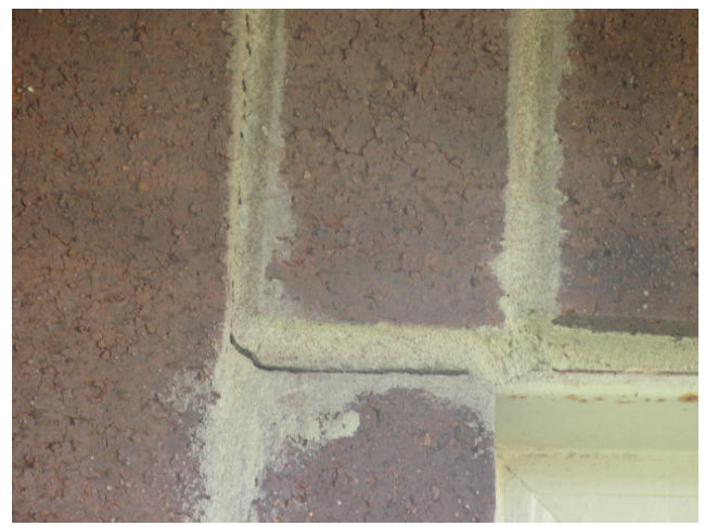
NOTED MORTAR JOINT CRACK
