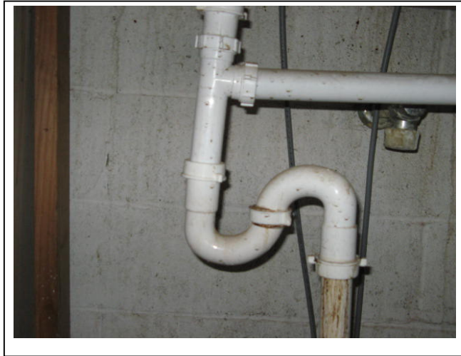
NOTED IMPROPER S-TRAP
