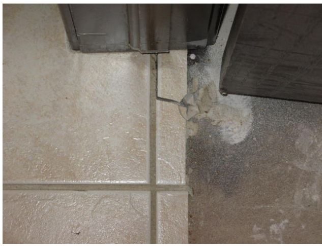
BROKEN FLOOR TILE
