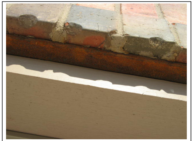
RUSTING STEEL LINTEL NEEDING PAINTED
