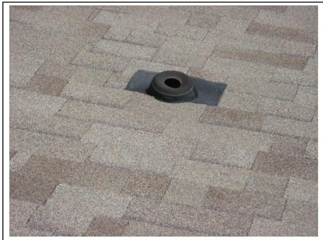
ROOF JACK WITH NO VENT STACK EXTENDED THROUGH THE ROOF
