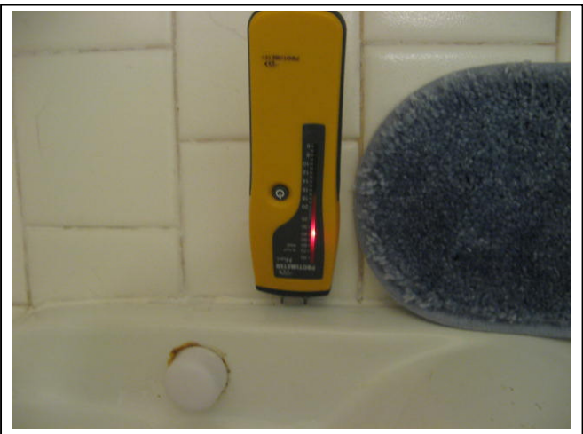
MOISTURE NOTED AROUND BASE OF STOOL.
